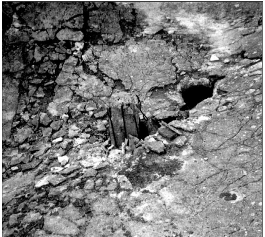
Document 8: Morgue 1 of crematorium II at Birkenau. Concrete pillar protruding from concrete roof slab and the crack produced by the pillar. August 2000. © Carlo Mattogno.
