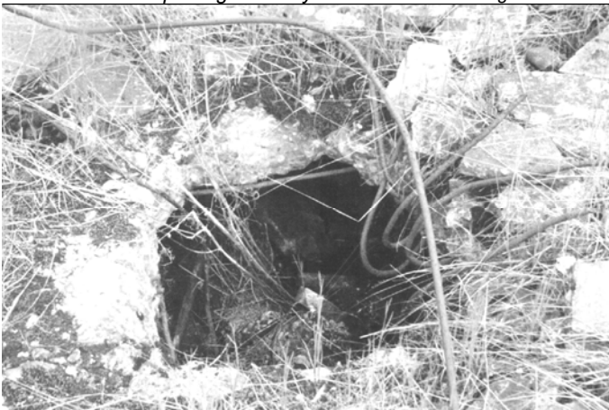
Photo 20: Concrete roof of morgue 1 of crematorium II in Birkenau. Opening 7 in June 1990.
