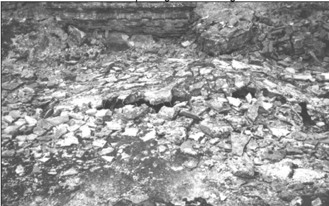
Photo 30: Concrete roof of morgue 1 of crematorium II in August 2000. Line of the crack, to which Provan's opening no. 8 belongs - to the right of this photo (see photo 31).
