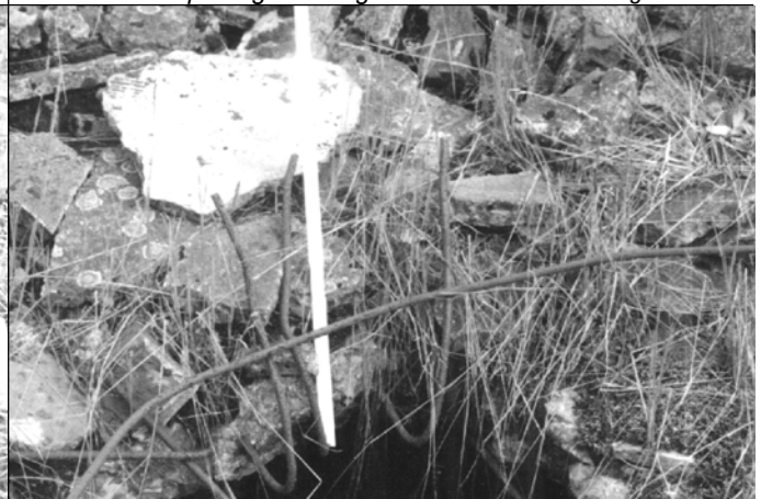
Photo 21: Concrete roof of morgue 1 of crematorium II in Birkenau. Reinforcement bars of opening 7 in June 1990.
