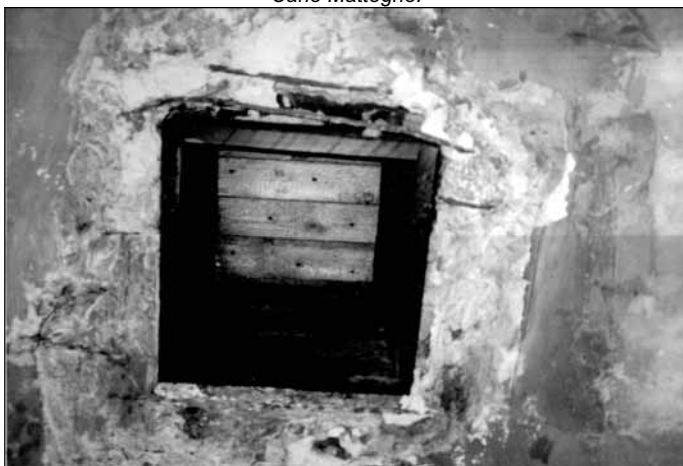
Document 13: Photo of the ceiling of the morgue. One of the four shafts constructed by the Poles after the war. © Carlo Mattogno.
