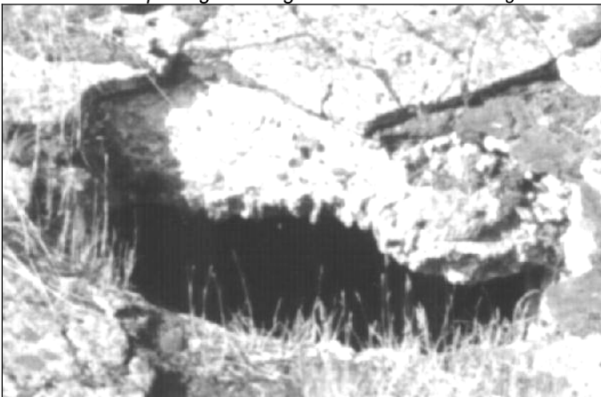
Photo 17: Concrete roof of morgue 1 of crematorium II in Birkenau. Opening 2 in July 1992. © Carlo Mattogno
