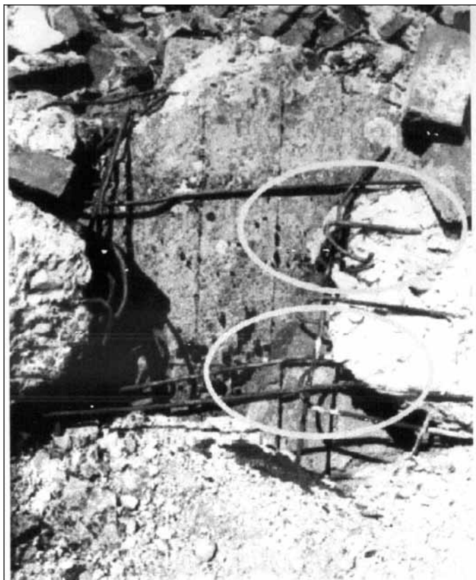
Figure 16. Remains of fourth (seen from south) Zyklon hole. Rebar skirts two sides, ends at other two sides bent inward and looped back. Note rotated roof slab showing formwork on inner side.
