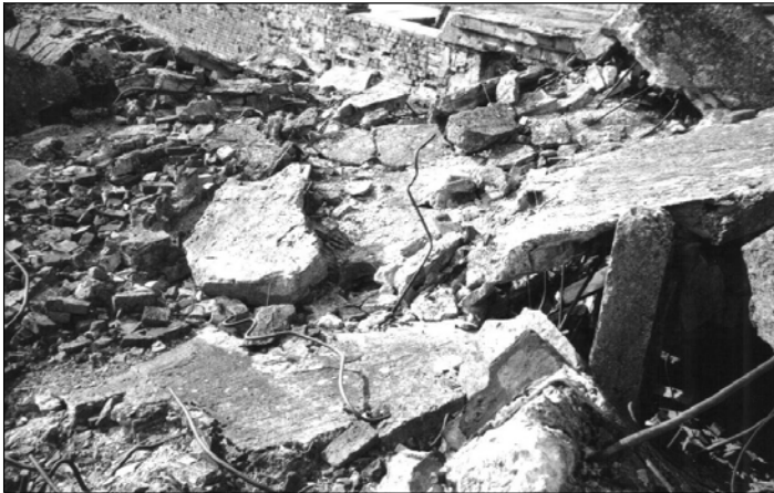
Photo 6: Round opening for the pipe of the ventilation through the reinforced concrete roof of morgue 2 of crematorium II in Birkenau. August 2000. © Carlo Mattogno.
